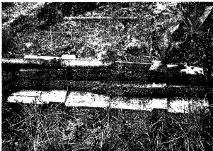
NO. 11.—CABLE SECTIONS INVOLVED IN FIRE SHOWING DEGREES OF DAMAGE.
